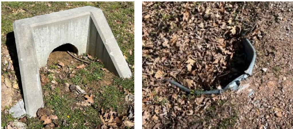
Figure 8: Existing Pipe Blockages
